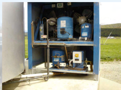
The Mahana Blue heat pump installed beneath the milk vat chiller unit at Glencairn
